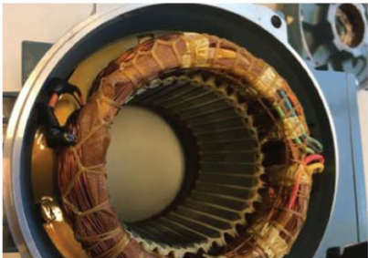
(b) stator-turn fault
